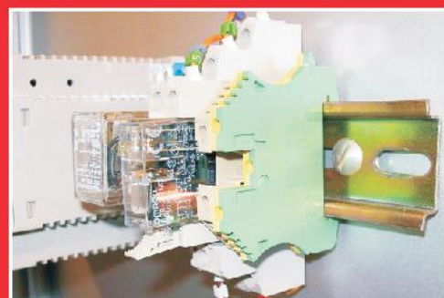
Electrical equipment is mounted onto 35 mm DIN rail
